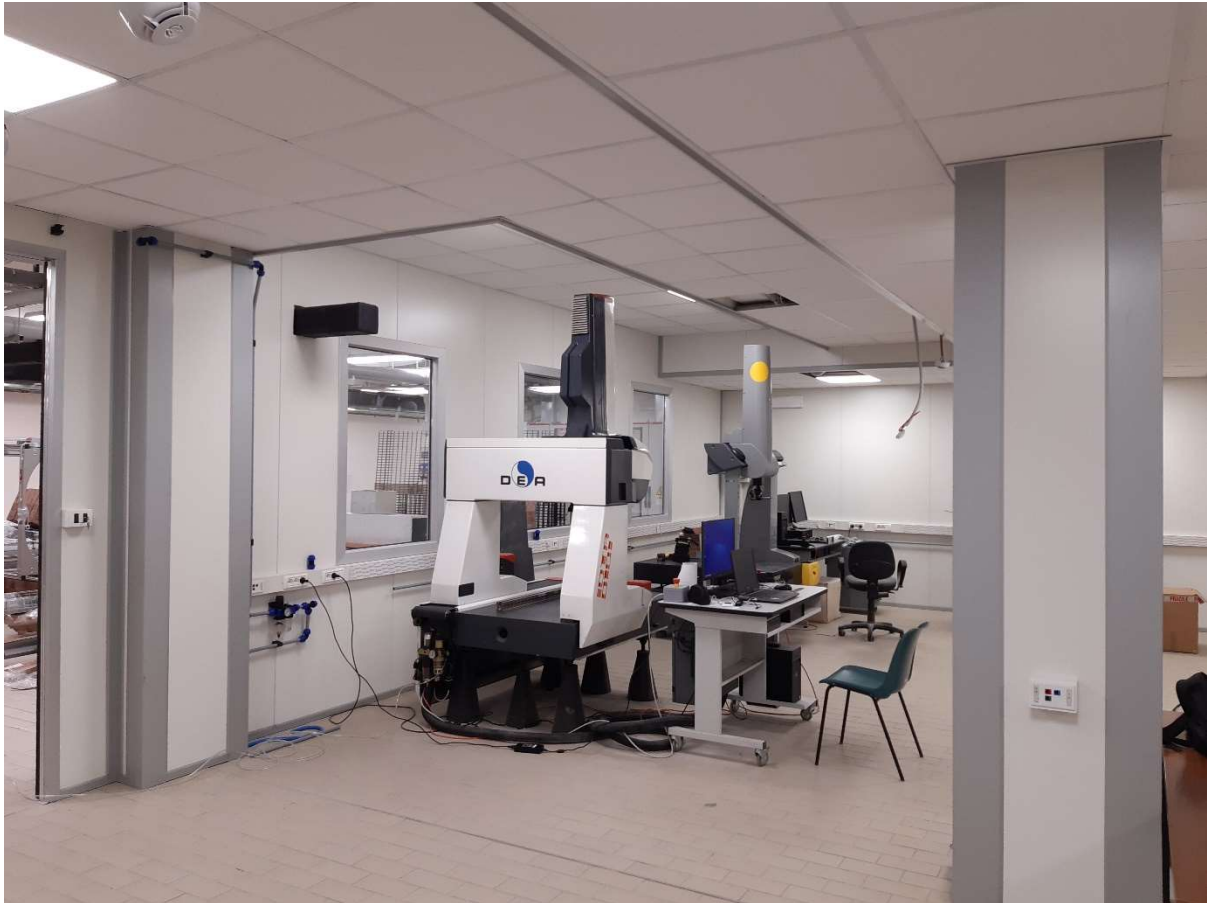
Figure F.1. Finalization phase of the construction of the new metrology cabin within the MInd4Lab.
